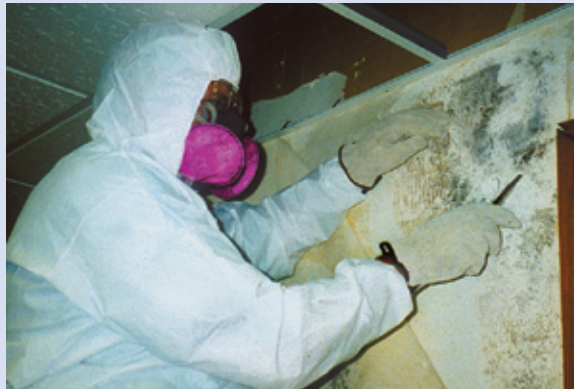
Photo 7: Remediation worker with limited PPE
